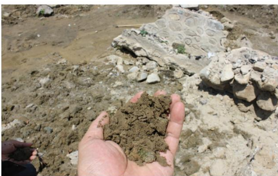
Figure 17. Loose – Very Loose Soils (Darjanto, 2018).
